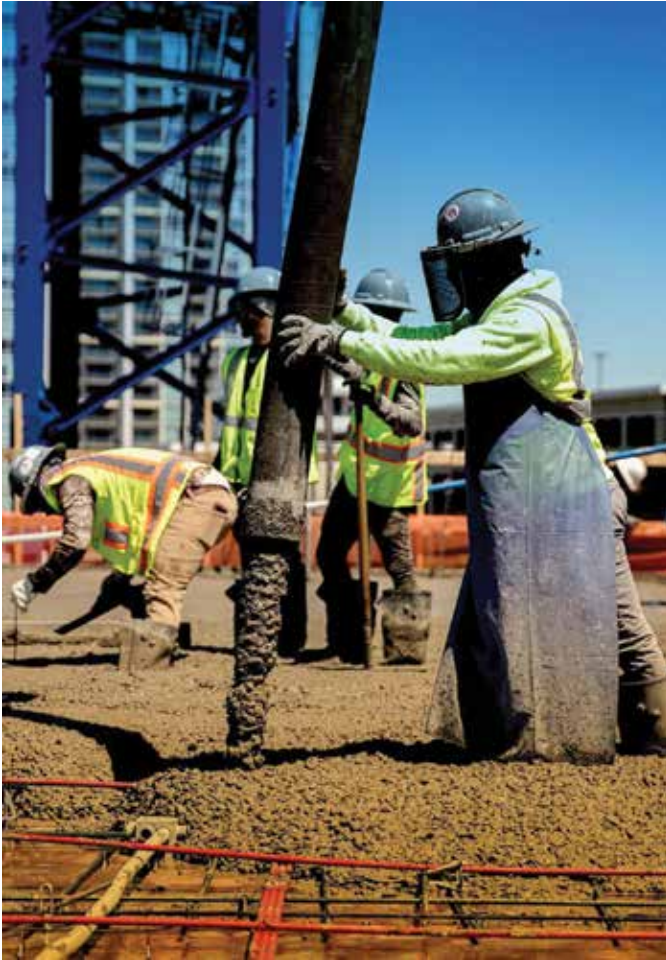
Baker Concrete is collaborating on cost-effective strategies for producing and placing more sustainable concrete
