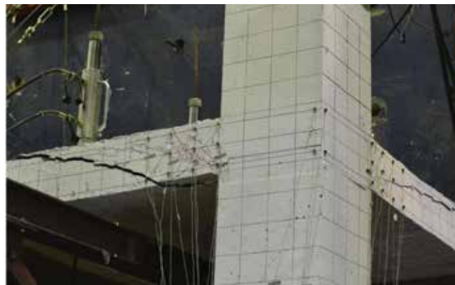
Crack pattern in corner slab-column connection at 1.25% drift (Fig. 4.43 from Final Report to the ACI Foundation: CRC 80)
