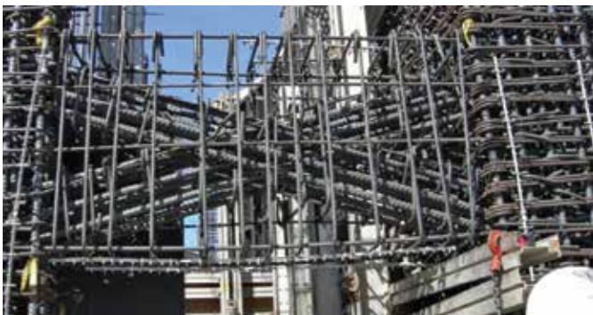
Example of a traditional coupling beam with “woven” diagonal bars and transverse reinforcement
